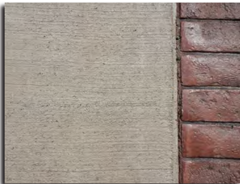
New Brick Soldier Course Plain Concrete / Dark Red Hardener Deep Charcoal Release
